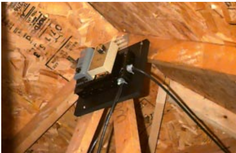
Ridge ventilator temperature & humidity control.
