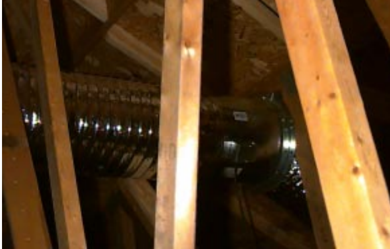
Ridge ventilator in-line blower unit.
