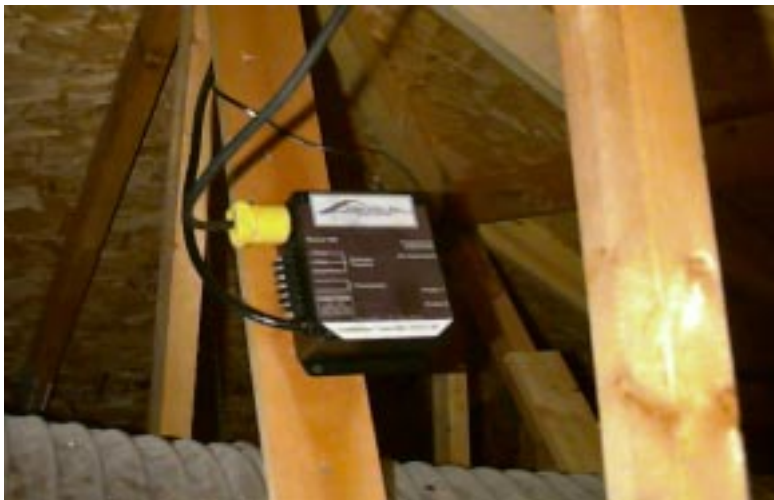
SAVC02 temperature & humidity control.
