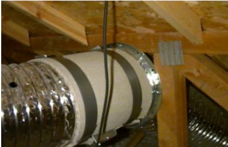
Ridge ventilator in-line blower unit.
